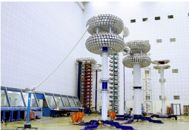
Calibration of DC measuring system 1000 kV
